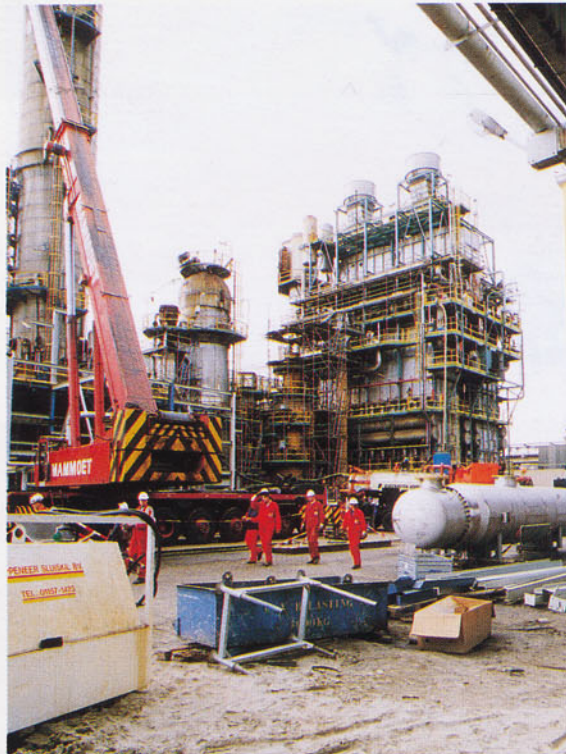
Sluiskil — Mammoet Stoof Terneuzen co-ordinated a large quantity of cranaage for the revamp and shut-down of an ammonia plant at Hydro Agri at Sluiskil. One of the highlights of the job was the installation of a reactor vessel which had been shipped from Japan by Mammoet Shipping. The ammonia plant, originally built in 1971, is now up to date again in terms of energy efficiency and environmental demands.
