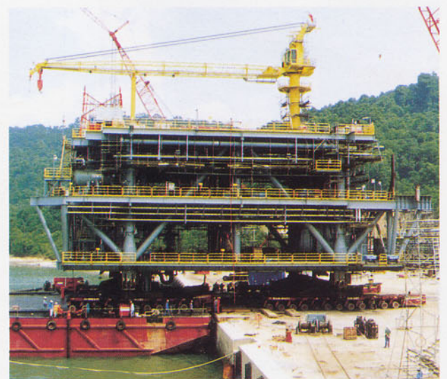
Penang — Walter Wright Mammoet's self-propelled modular transporters were used for several load-out operations for the offshore industrie at Penang in Malaysia. The picture shows a 1,100 tonne riser deck rolled on to an ocean going barge.
