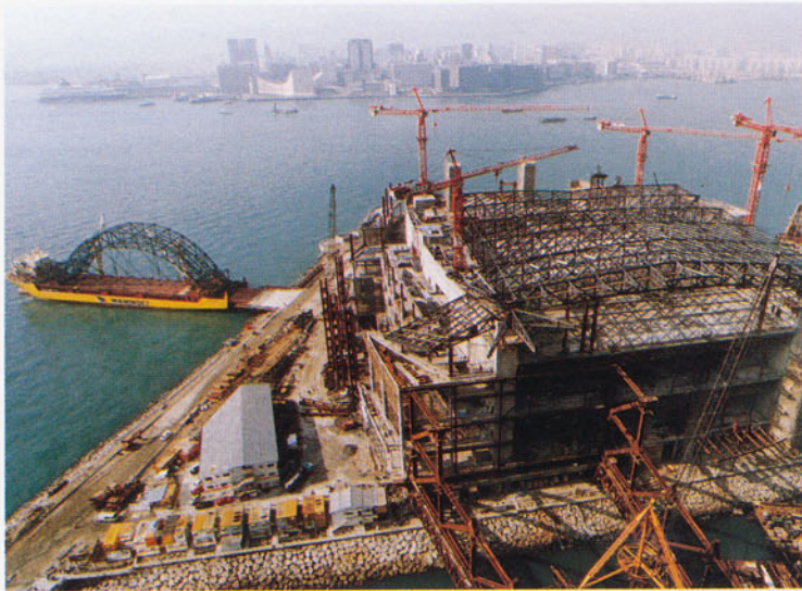
Hong Kong — A huge bird-shaped steel and glass structure is built at the Wan Chai waterfront which is part of an extension to the Hong Kong Convention and Exhibition Centre. One of the last roof trusses was delivered by Mammoet Shipping's "Thor Scan". The extension will double the size of the centre.
